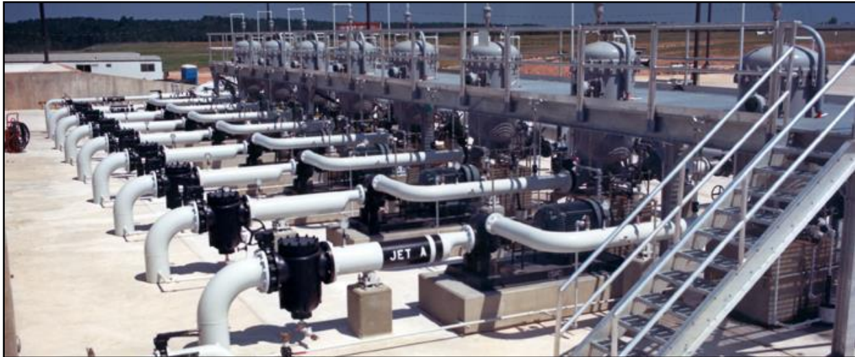
Figure 1. Pump station that uses vertical pumps to transport jet fuel from underground storage tanks to the airport [5]. Note that the text size of the caption is smaller (10 points) than the size in the main text. Also, the line spacing is 1.0 spacing. Such a difference serves to separate the caption text from the body text. Finally, note the vertical space given before the image and after the caption.
